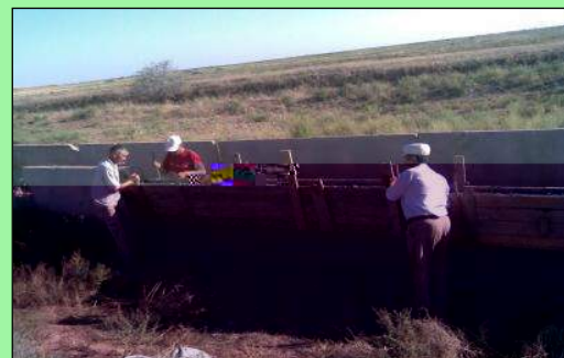
Figure 1. Reconstruction of irrigation canal by local community for autumn and early-spring irrigation of alfalfa from the Talas River (Photo by: Gulnara Bekturova)
