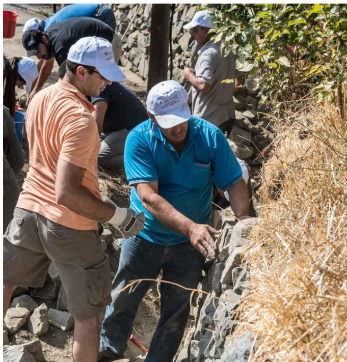
Stakeholders restore collapsed dry-stone terrace walls following instructions given by experts. (Christos Zoumidis)
