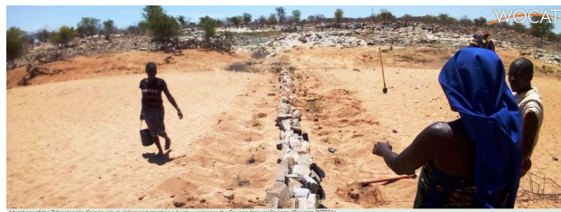
Members of the Tchikongolo Community building and planting a Leaky well near the Caungo Natural Springs. (Project RETSA)
